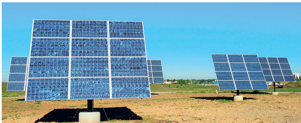
Solar energy panels
