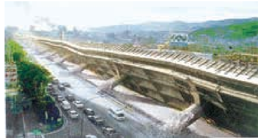
Aftermath of an earthquake .
